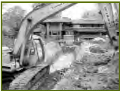
The excavation for the pergola's foundation. Courtesy of the Martin House Restoration Corporation.
